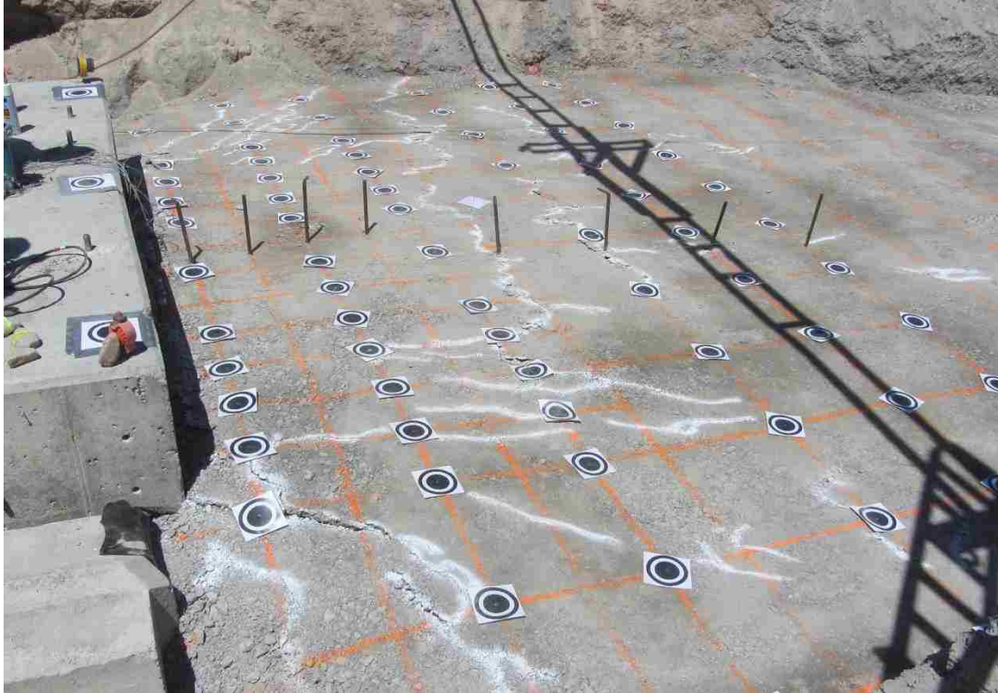
Figure 4-28. Backfill surface at end of non-skewed 3.5 ft (1.07 m) gravel test, viewed from the east side.
