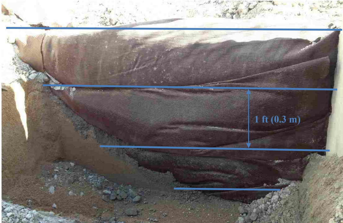
Figure 3-14. Geotextile fabric layer folds along the front of the backfill, made visible by removing the west transverse wingwall after testing.
