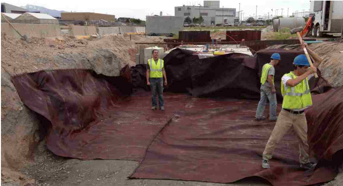
Figure 3-12. Every 1 ft (0.30 m), a new layer of geofabric reinforcement was placed in the backfill area. Overlap of the two sheets of fabric is visible in the top middle of the photo.
