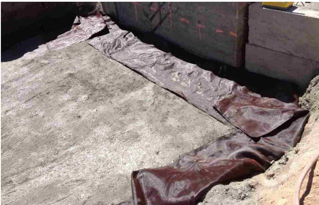
Figure 3-13. Extra geofabric was folded over the 1-ft (0.30-m) gravel layer in the non-skewed GRS test before placement of the next fabric sheet.
